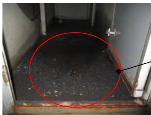
Sludge on floor surface
