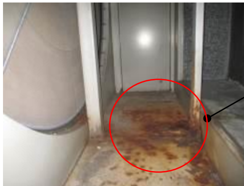
Rust on floor surface
