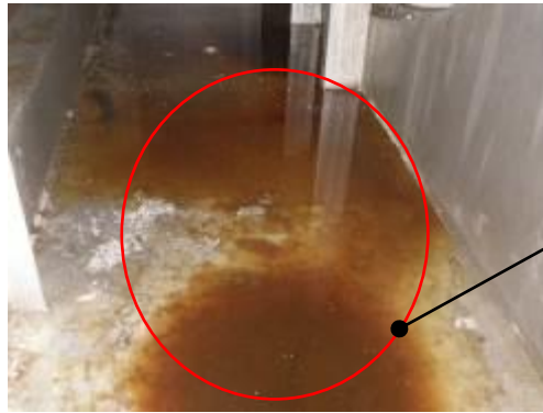
Liquid on floor surface
