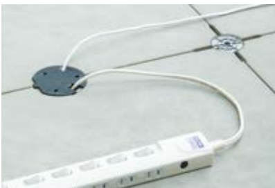
LAN cable + multi-tap outlet
