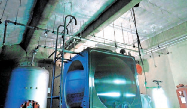
Mechanical room : Heat & Sound insulation
